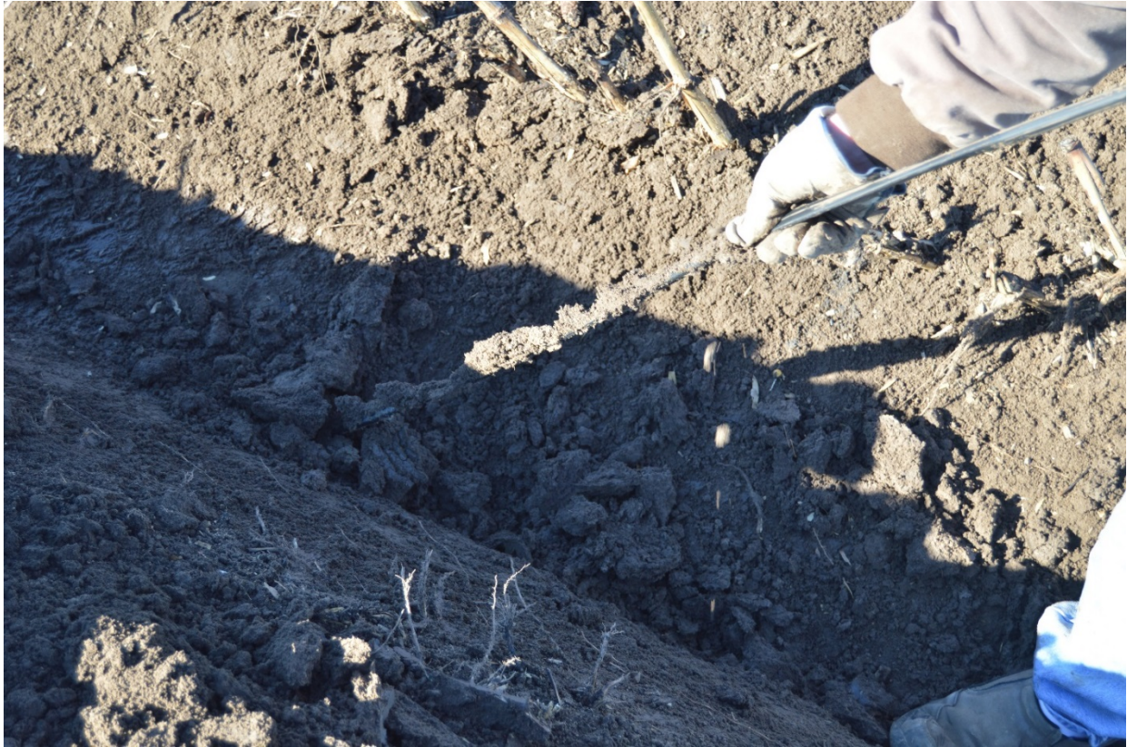
Figure 5. Careful extrication of the dripline from the remaining 5 to 7 cm of soil overburden.
