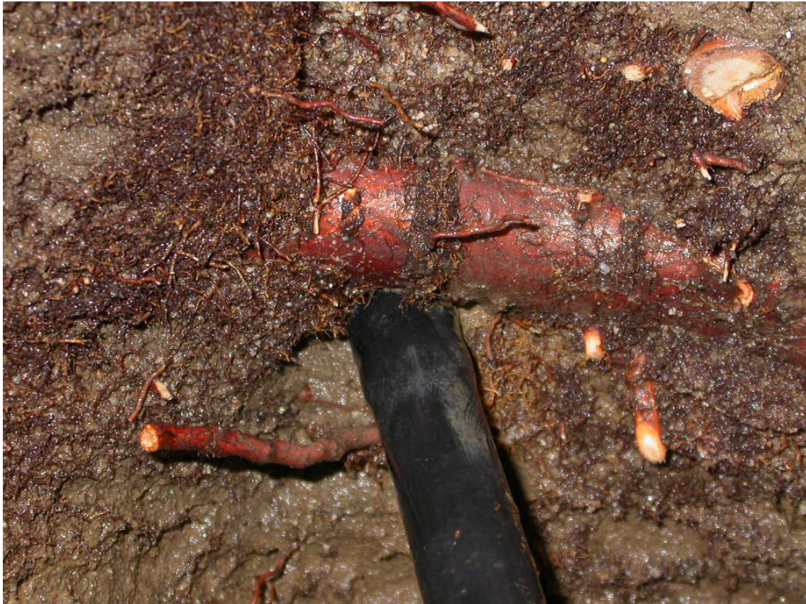
Figure 7. Subsurface dripline pinched by peach tree root in California, USA. Photo courtesy of T. Trout, USDA-ARS, Parlier, California.
