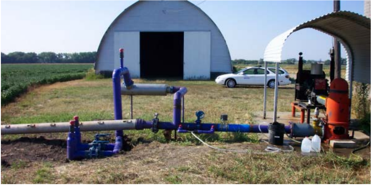
Figure 3b. Improved pumping plant and filtration configuration of the case study SDI system.
