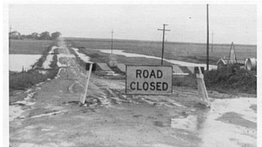
View of runoff from rangeland south of NWREC after a severe thunderstorm on July 13, 1989.
